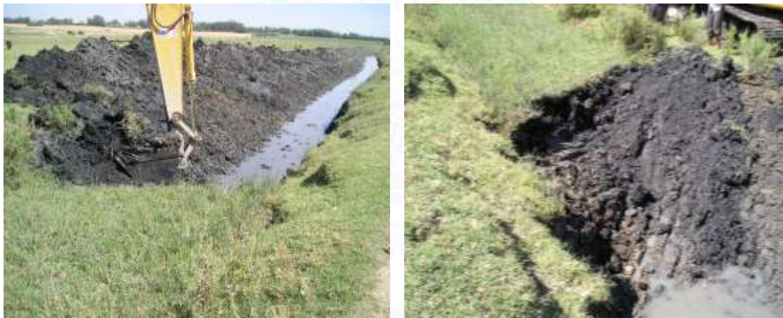
Figure 1. The appearance of the channels of the collector-drainage system after the annual drying out and formation of a blockage due to the formation of vegetation
